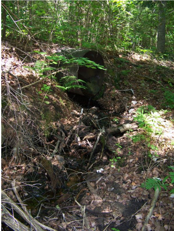
Figure 12: Stream 2 flowing through breached culvert beneath road allowance
